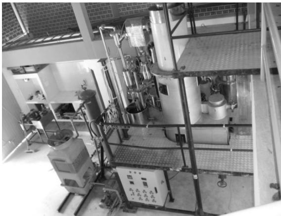
Figure 1. The imported open top biomass gasifier.
