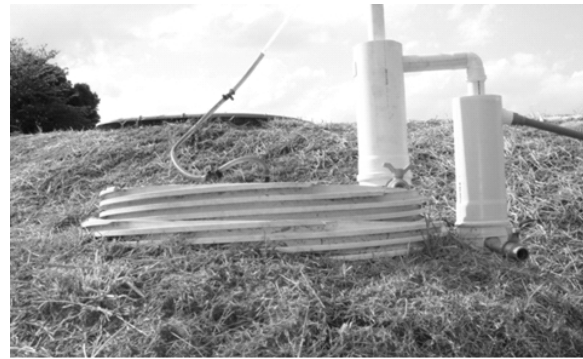
Figure 6. Filtration system installed in gasometre.
