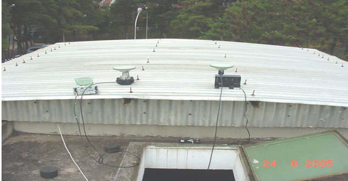
Figure 1 - The antennas at the EESC – USP Campus and the rover antenna is mounted over the EMO.
